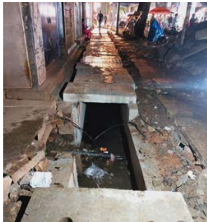
Unfinished drainage work
