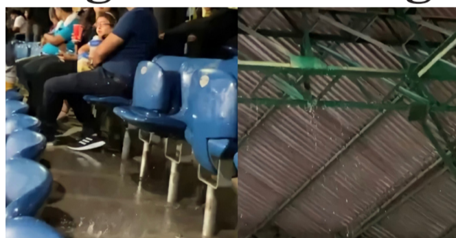
A leak in the roof at the stadium
